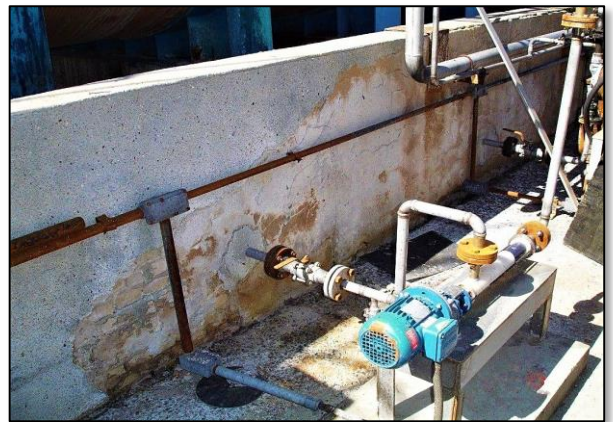
Pumping of sulfuric acid in a plant
