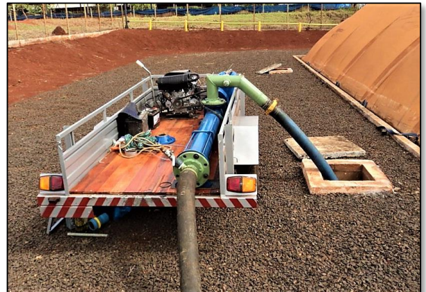
Pump with diesel engine
